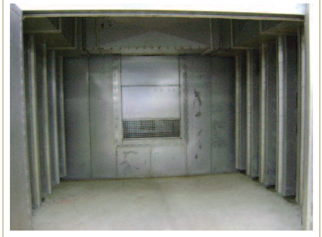
Typical electric convection batch oven 300kW
